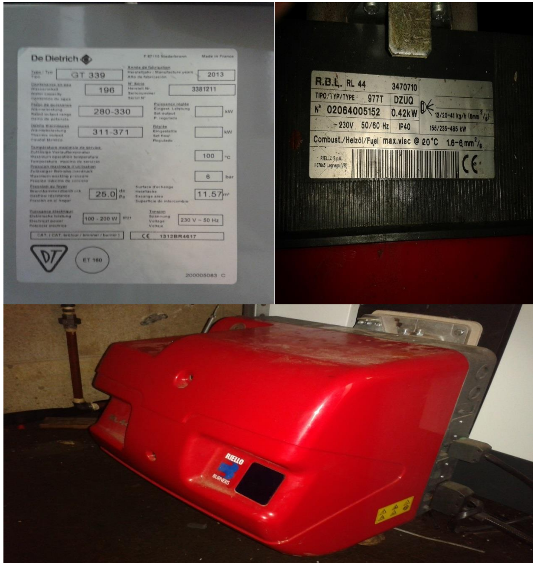
Figure 5 Boiler/Burner ID plates and Burner
