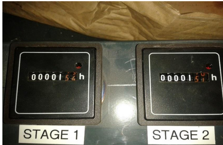
Figure 9 Burner On-Time for both Riello burners.
