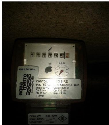
Figure 8 Oil Volume meter
