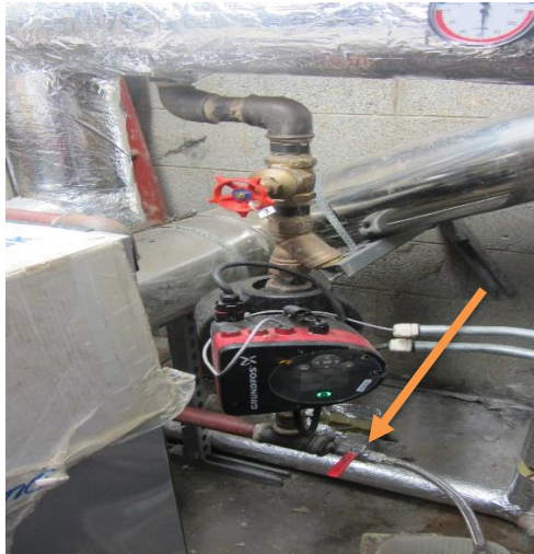
Figure 7 Sample drain valve.
